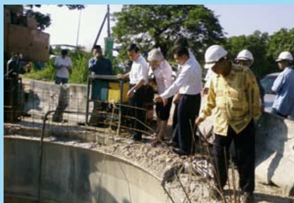
Penang State Exco YB Lim Hock Seng, Bukit Mertajam Member of Parliament YB Chong Eng and Padang Lalang State Assemblyman YB Tan Cheong Heng visiting the site of Juru Sewage Treatment Plant Project in Taman Kota Permai, Bukit Mertajam. The project by Jabatan Perkhidmatan Pembetungan (JPP) was started in 2007. It has received numerous complaints from nearby residents regarding the effect of the construction to their homes. Through the efforts by the State Government, YB Chong Eng and YB Tan Cheong Heng, residents are assured that damages to their homes due to the project will be compensated by the project contractor.
