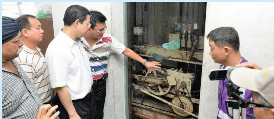
Lift maintenance company staff (fourth from left), showing CM Lim (on his right), the faulty lift system at the engine room. Looking on is Chairman of the Management Committee, Chuah Boon Kwan.
