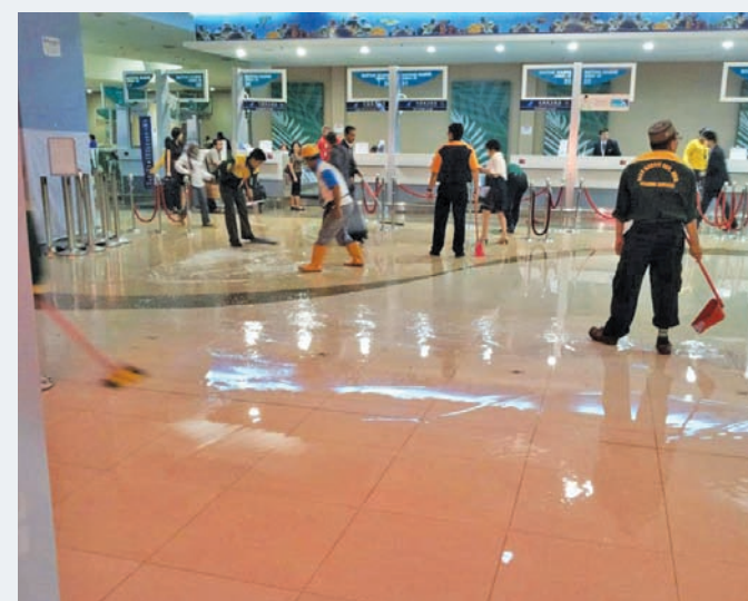
This photo taken by an airport user was sent to the Chief Minister's office. Water gushed down from the ceiling in what was described by the user as 'water flowing like a waterfall' while airport workers tried frantically to mop it up.
