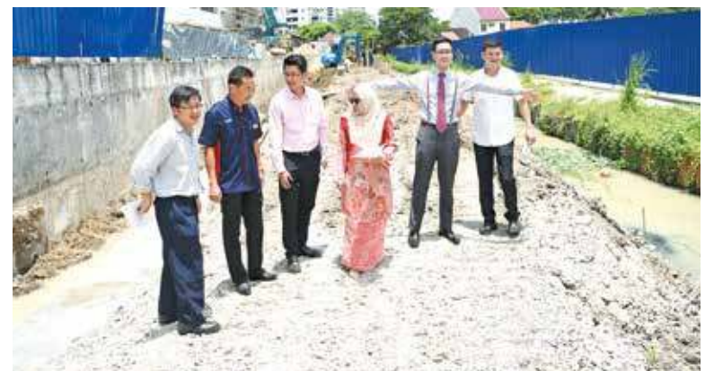
Zairil (second from right) showing the area which will be involved in the Sungai Jelutong flood mitigation project.
